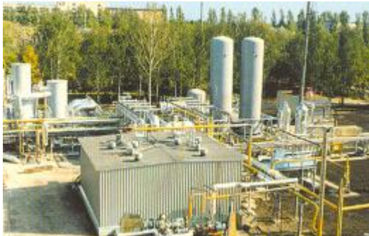
Gas Reducing Stations
