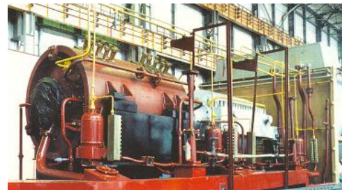
Complex gas treatment plants
